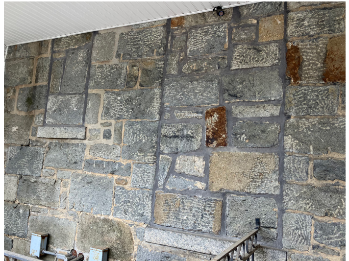
32. Not Recommended: Poor mortar and infill.
