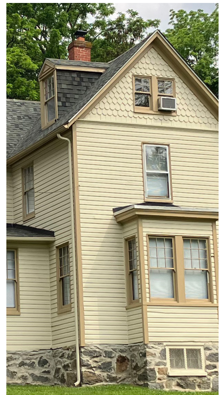
33. Gutters and downspouts should direct water away from the building to prevent rainwater accumulation and penetration at the building's base.
